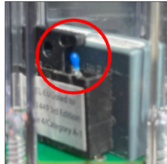
Normal Operating Condition: Blue flag under hood
