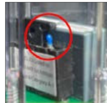
Normal Operating Condition: Blue flag under hood
